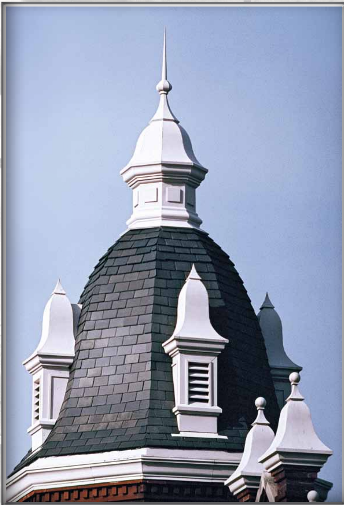
Copper finials and dormers adorn Temple B'Nai Shalom in Huntsville, Alabama. The architectural ornaments were painted white for historical accuracy.
